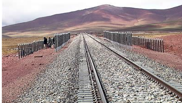
Figure 2: Volume problem of crushed stone in the roadbed of Qingzang Railway
