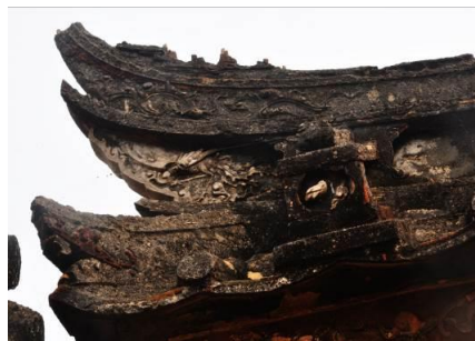
Figure 16: Gray molding decoration on the ridge of the roof in Chaoxi Village (Source: Self-portrait)
