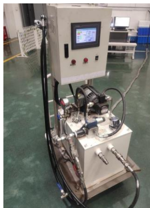
Figure 4: Fuel oil supply unit
