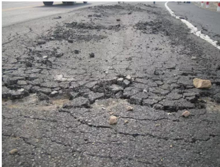
Figure 3: Uneven road surface.
