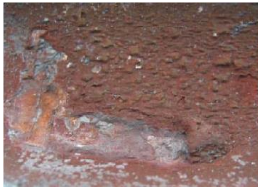
Figure 5: Morphology of pipe metal substrate after removal of corrosion products on inner surface.
