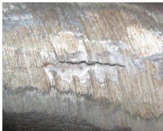
Figure 3: Appearance of crack-like bursting port.
