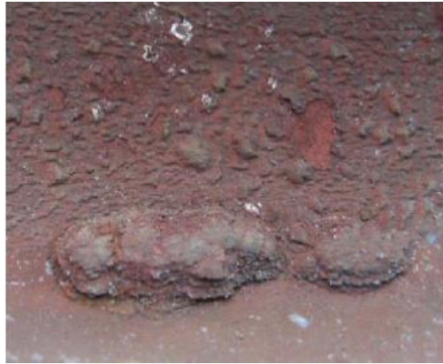
Figure 4: Inner surface near the crack-like bursting port.
