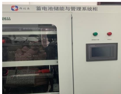
Figure 4 Battery energy storage and management system cabinet
