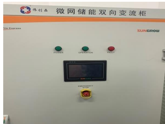
Figure 6 Microgrid energy storage bidirectional converter cabinet
