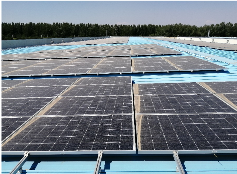
Figure 1: Photo of the dust belt on the lower frame of the solar module
