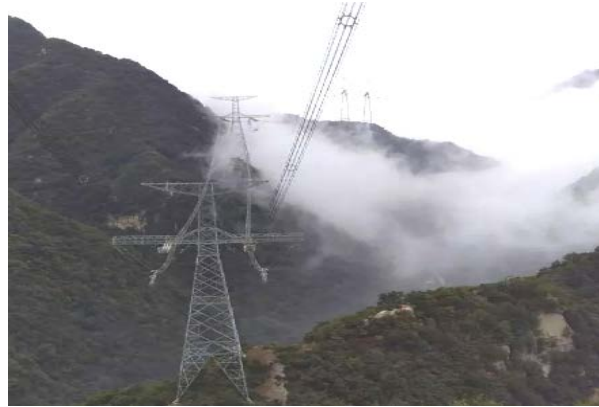
Fig.1. UHV transmission line in plateau areas
